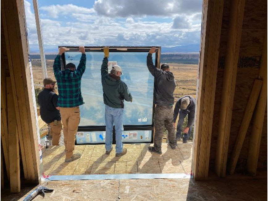
Heavy lift. It took five guys to muscle one of the living room wall windows into place.
