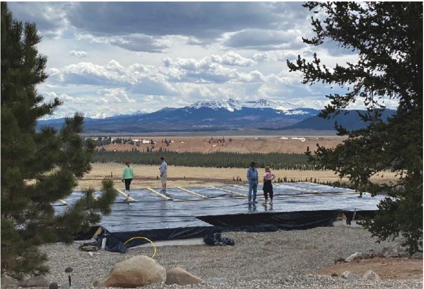
John, our contractor, stands in the future kitchen with Terry while Brenda and Andy imagine the view from the living room.
